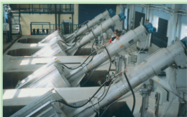
Stainless steel rotary drum fine screens with integrated screenings washing installed in parallel (Photo: HUBER SE, Berching, Germany)
