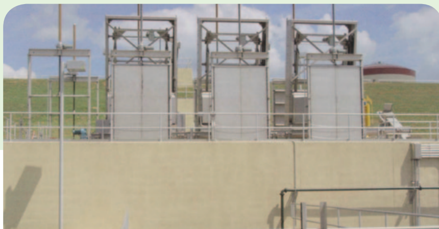
Stainless steel slide gates between two wastewater basins (Photo: Nickel Institute, Toronto, Canada)
