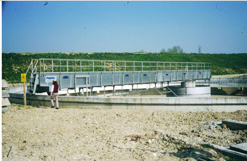
Figure 8 (March 1994) - Primary and secondary sedimentation. The rotating stainless steel bridge installed in each circular tank
