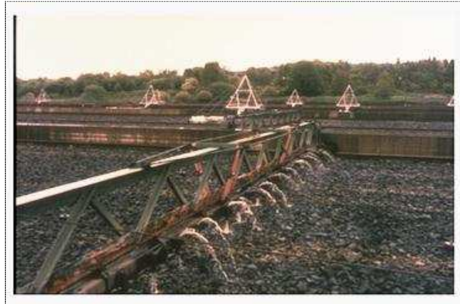
Figure 5. Heaton Lodge, UK. Coated steel distributors in the foreground have been replaced with new a pyramid shaped design made from type 304 and 316 stainless steel as shown in the background.
