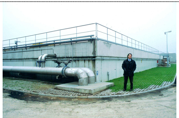
Figure 7 (March 2001). Pipe work to convey air for the Biological Oxidation . In the foreground a pair of stainless steel collectors, 700 mm diameter.
