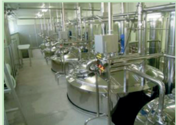
Multi-process tank (Narasaki Sangyo Co., Ltd.)
