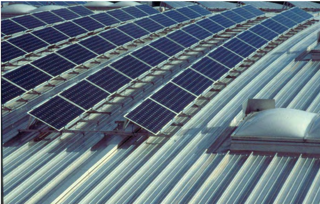
Fig. 35: Support devices for photovoltaic modules on flat metal roof (Messe München, hwp).
