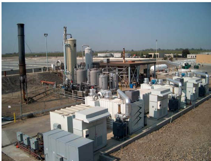
Figure 16: FuelCell Energy facility at the Tulare, California Wastewater Treatment Plant. Photo courtesy of FuelCell Energy, Inc., NREL/PIX 19193
